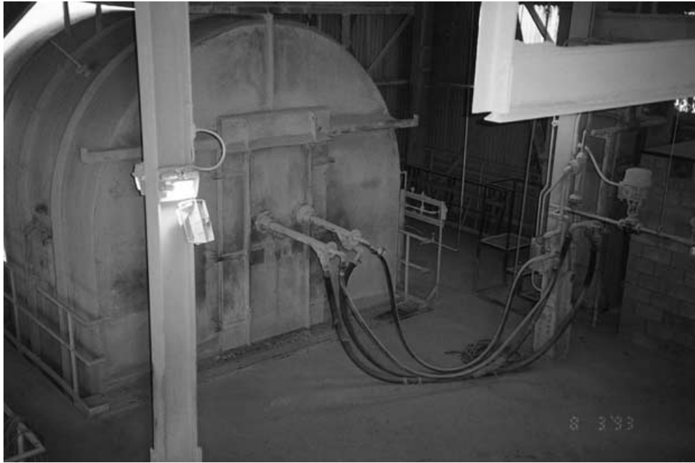
Figure 12.10 Kiln header box with water injection cooling lances (2) (center of photo with water supply hoses attached).
