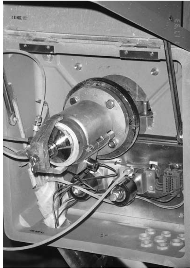
Figure 12.7 Sample probe protection box (interior view) with sample probe heated filter (center). Integrally heat-traced-and-insulated process sample transfer line exits sample probe protection box from lower-left bottom of box.
