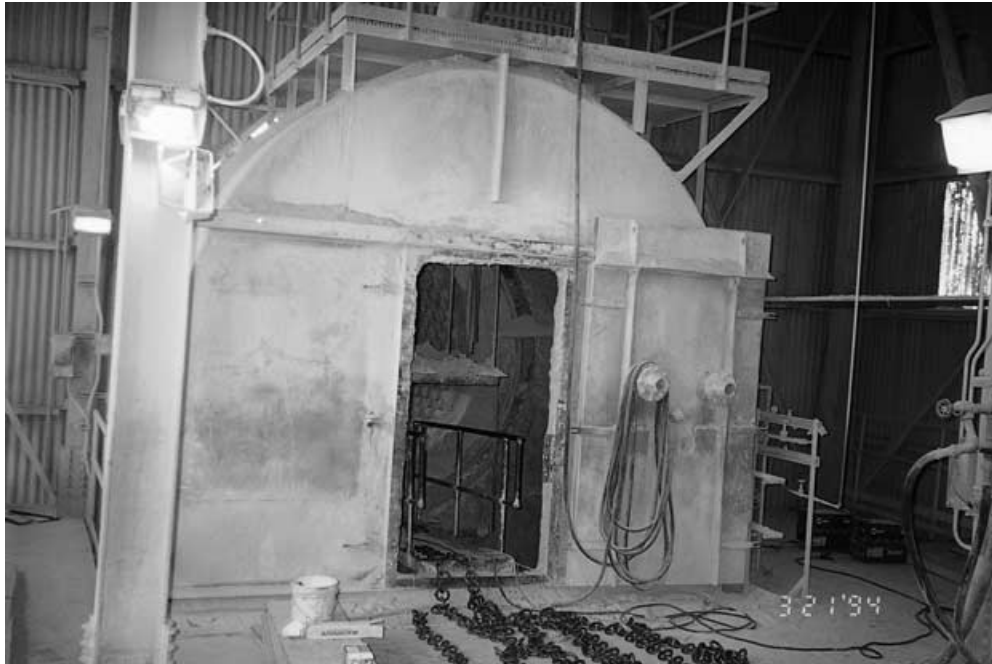
Figure 12.11 Kiln header box access door (open) showing internal support structure and water injection cooling lance (internal connections).
