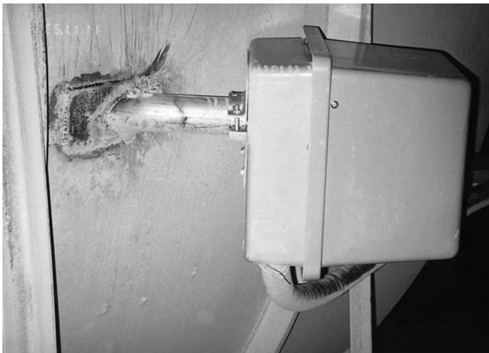
Figure 12.5 View of process analyzer sample probe showing kiln header box exterior wall penetration detail and sample probe protection box detail. Integrally heat-traced-and-insulated process sample transfer line exits sample probe protection box from bottom of box.
