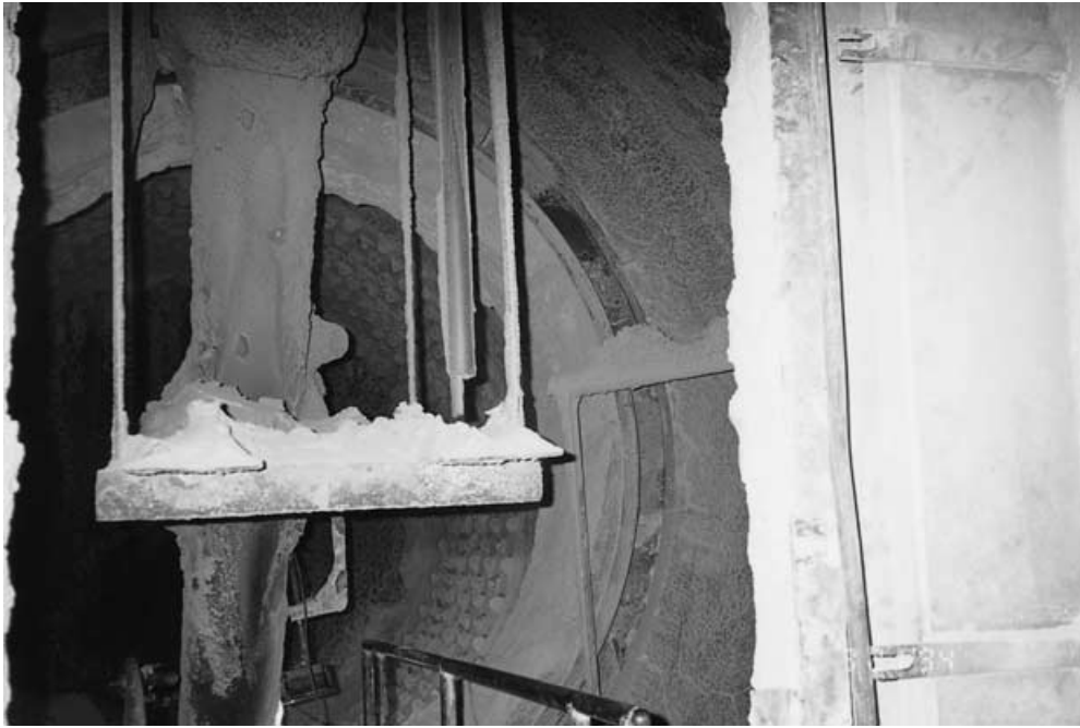
Figure 12.8 Kiln interior showing water injection cooling lance in lower right (below probe support).
