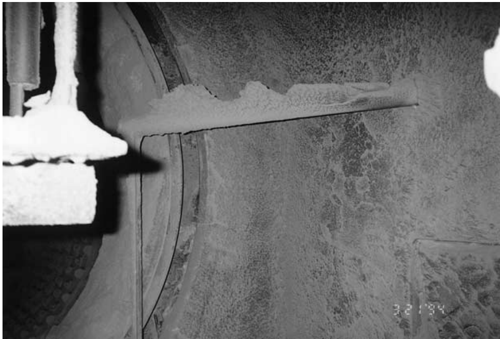
Figure 12.4 Rear view of supported process analyzer sample probe showing process material build up (residual) and sample probe kiln header box penetration.
